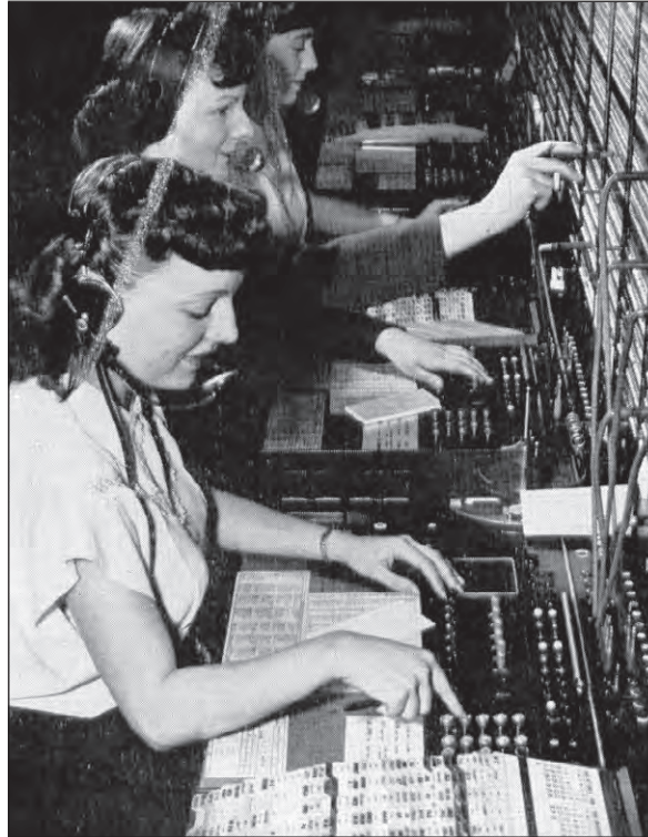
Toll switchboard in New York City showing push button dials at each position.
